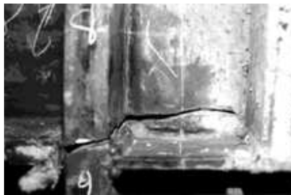
Figure 1.1: Fracture in welded steel beam-column joint [16]
